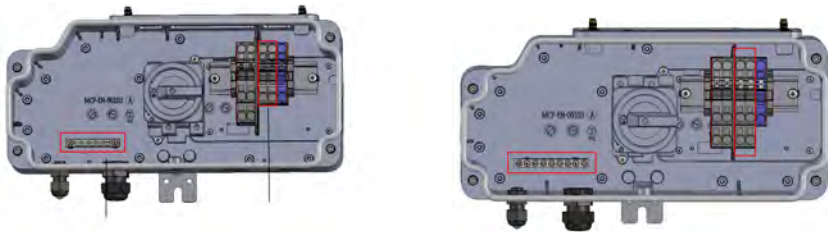
Figure 7: Inside the DC Safety Unit before (left) and after (right) replacements
